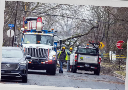
Modernizing our energy infrastructure
